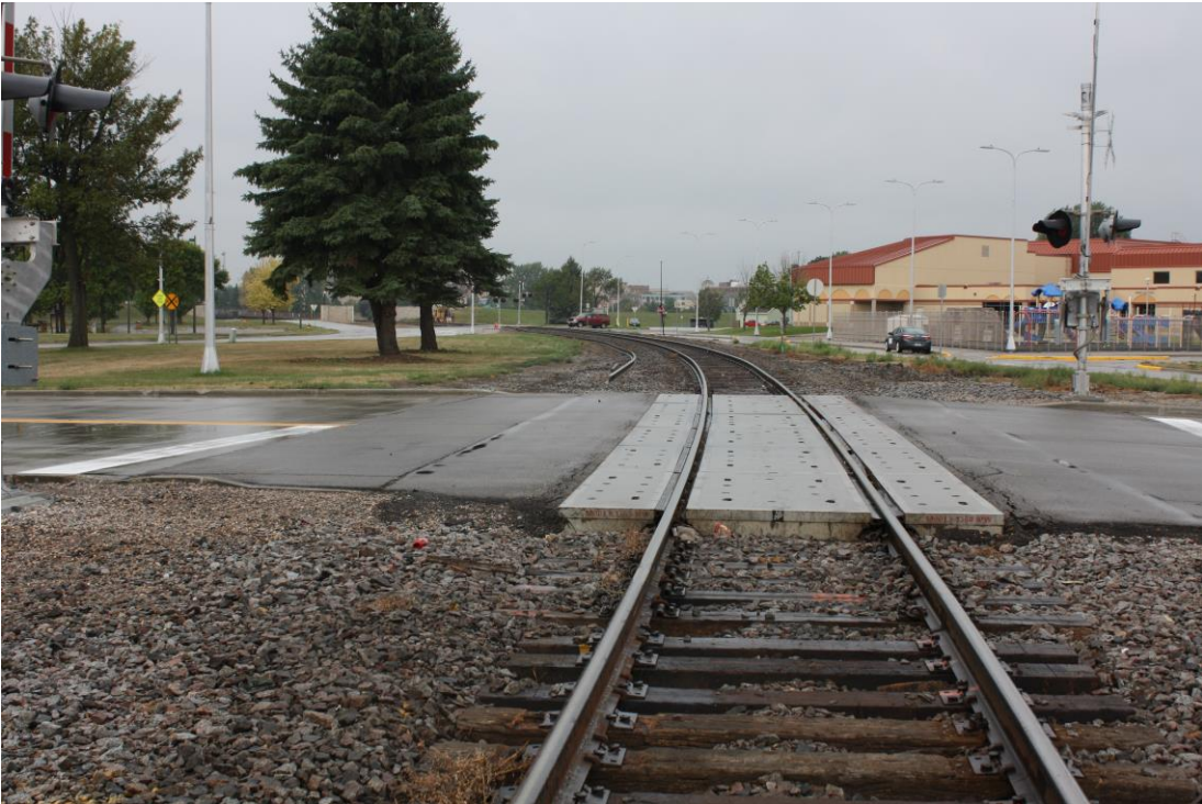
Multi-modal Rail crossing Near School Center – East Grand Forks, Photo: © MPO Staff, 2017
