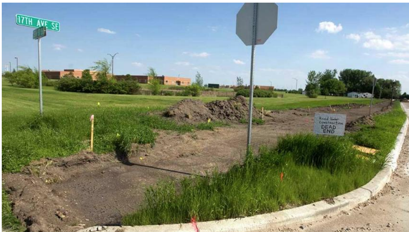
A sidewalk is under construction along 17th Avenue SE and 13th Street SE in East Grand Forks last week. Grand Forks Herald photo by Sarah Kolberg. (June 12, 2010)
